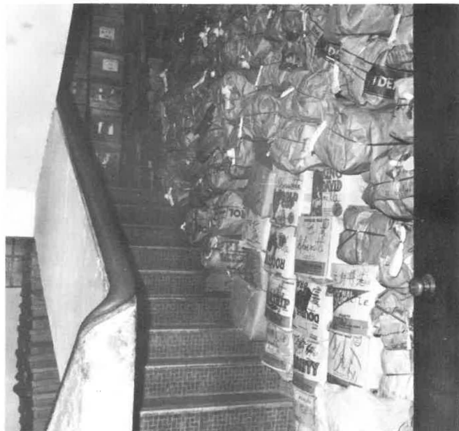
The staircase, often the only storage area for a factory in domestic premises, and also the only escape from a fire.
